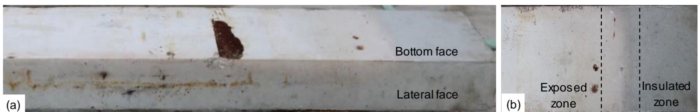
Fig. 8 – Appearance of slab Fire 60 – 1 after exposure to fire: (a) Overview of the bottom and lateral surfaces of the slab; (b) Intermediate zone of the bottom surface of the slab, between the exposed zone and the unexposed zone.
